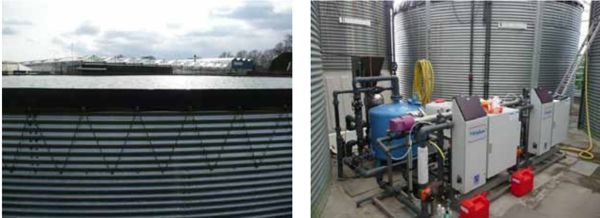
Figure 3.4 Rainwater collection tanks or basins are mainly located outside, but all other storage tanks stand inside the glasshouse. At the right picture at the foreground the disinfection installation (UV radiation) and the blue rapid sand filter. The tanks at the background are for collecting water to be disinfected “dirty water tank” (right) and for waste water to be emitted to the sewage system.
