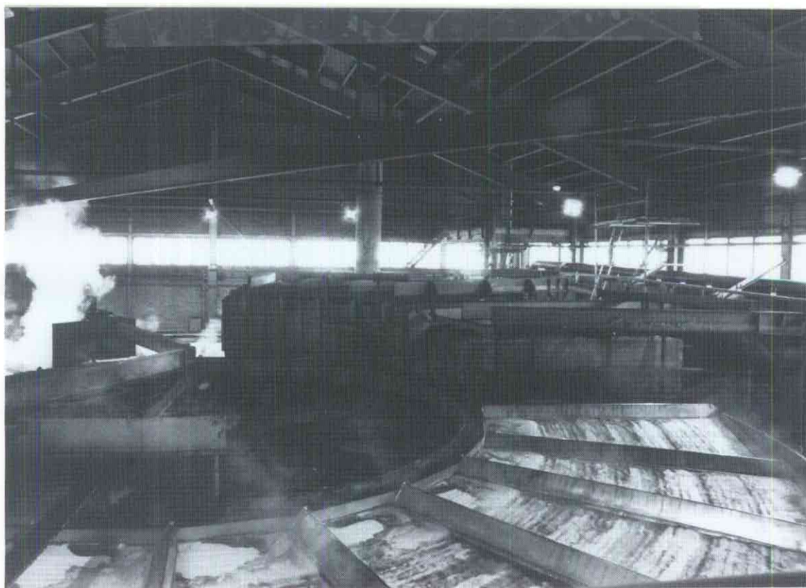
Filter system (about 200 m 2 ) for the processing of phosphate ore intended for the manufacture of phosphoric acid (Kemira Pernis BV, RIVM photograph)
